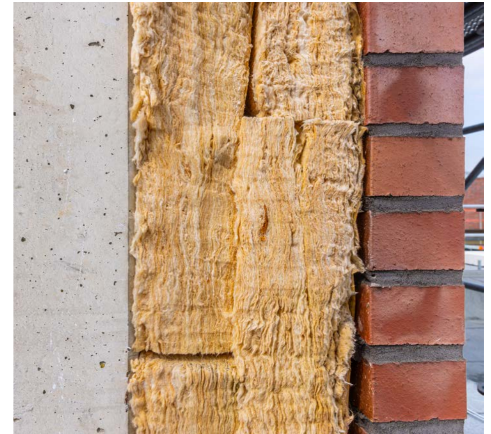
This image shows that the individual components of the wall construction can easily be separated into different types of material in the event of deconstruction.
